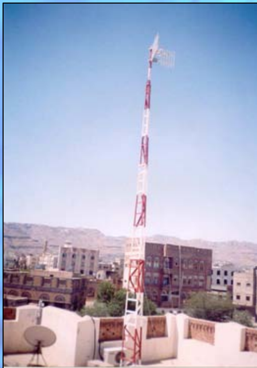
Line of Sight Survey work in Sana'a for Canadian Nexen (installing repeater towers).
